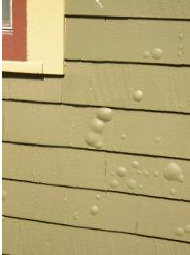
Slika 5. Mjehurenje premaza (Izvor: https://www.house-painting-info.com/articles/blistering/ )
