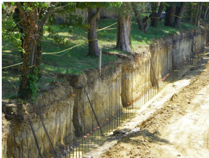
Slika 1. Rov iskopan tijekom građevinskih radova u neposrednoj blizini starijih urbanih stabala. (Izvor: Full circle tree & shrub L.L.C., Construction damage: How to Preserve Your Landscape https://fullcircletreeandshrub.com/blog/construction-damage-how-to-preserve-your-landscape/ (Pristupljeno: 18.9.2021.)
