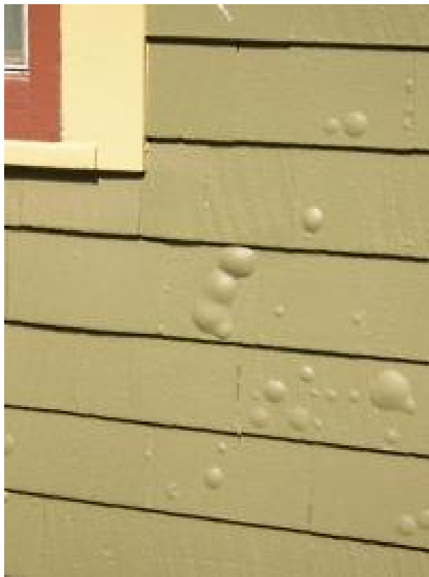
Slika 5. Mjehurenje premaza (Izvor: https://www.house-painting-info.com/articles/blistering/ )
